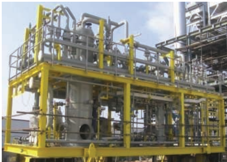
FIGURE 1. This photo shows a fluegas-conditioning module, which is part of a large process plant that was fully fabricated in a local shop in the Middle East to achieve the desired schedule
